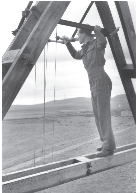
127 Leading Aircraftman L K Williams cleaning the feeder insulators on one of the 240 foot receiver towers at Saligo.
