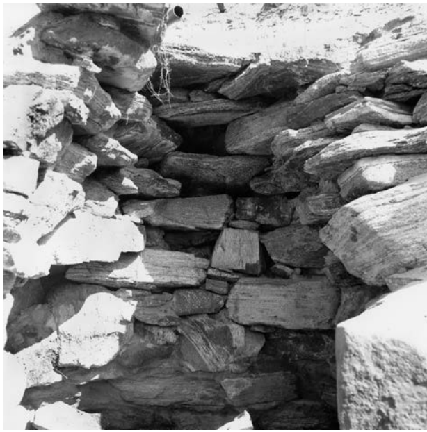
ILLUSTRATION 2.5 Detail of upper corbelling of Bay 4, looking up from the front of the bay.
