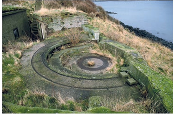
Figure 10.35 The southern of the two Second World War 6-pdr emplacements on Inchcolm, as it was in the 1990s (© Ron Morris)
