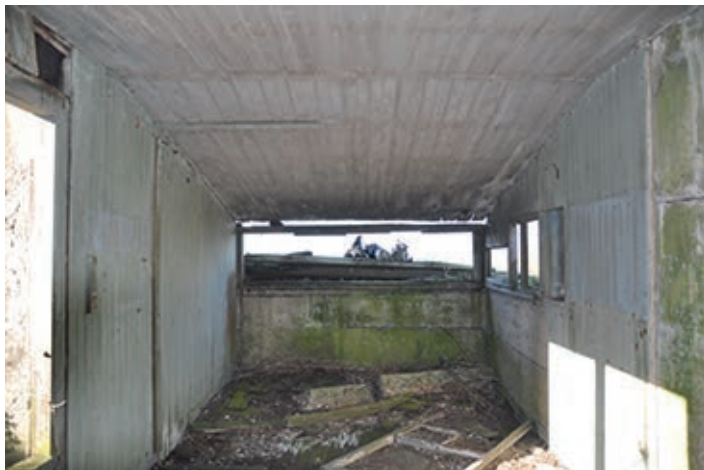
Figure 11.25 The western observation room of the former Fire Command (North) (© Gordon Barclay)
